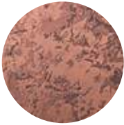
H8 DeErosion su rame DeErosion on copper
